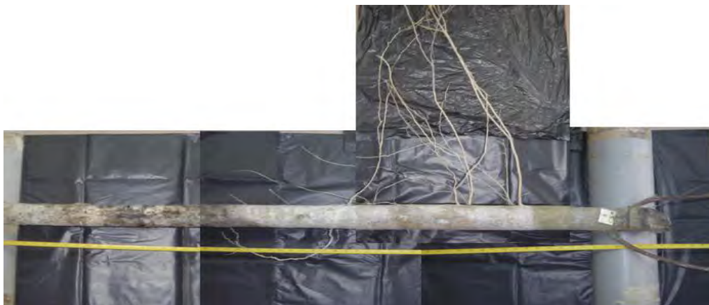
Figure 18: An exhumed Ht live pole
