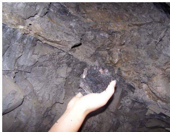
Figure 9: Surrounding rock mass condition of the central substation in the Hebi coal mine.
